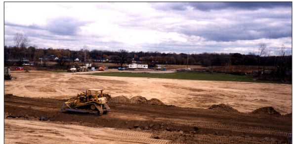
Construction of a soil cover (exposure barrier) over the former Linden Road Landfill in Flint Charter Township (Genesee Co.).
